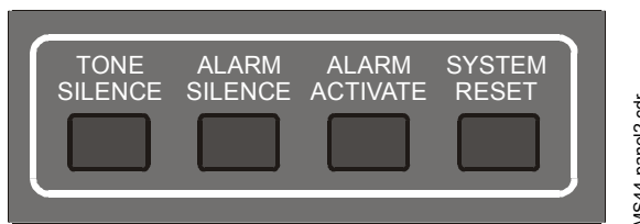
Figure 22 Control Panel Switches
